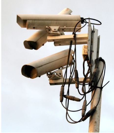
Figure 4 - 2 Surveillance using CCTV
